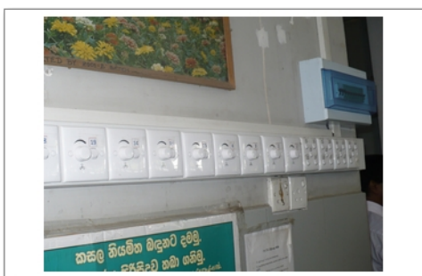
Repairing of Existing lamp fitting and ceiling fans and providing new electrical
