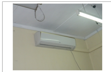
Air conditioner at the Ultra Sound Scanning room
