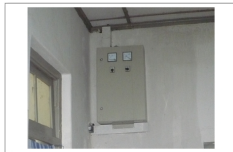
Power Distribution panel at the Laboratory
