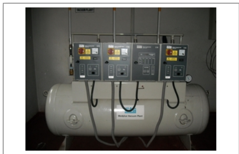
Increase the capacity of Medical Gas System) - 3.4 million
